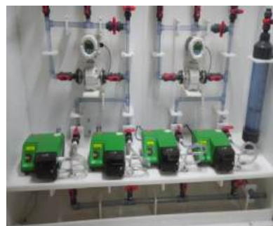
H_2O_2 Metering Pumps
