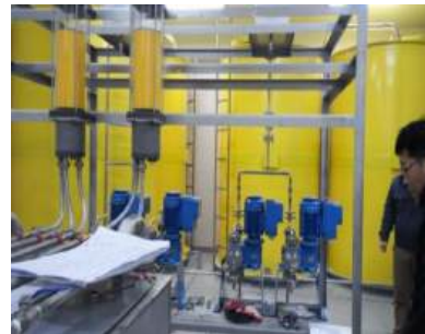
H_2O_2 Metering Pumps
