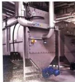
Horizontal wastewater 2x RoWin BCB Therm, extraction capacity 540 kW (wastewater) 900 kW (cooling)
